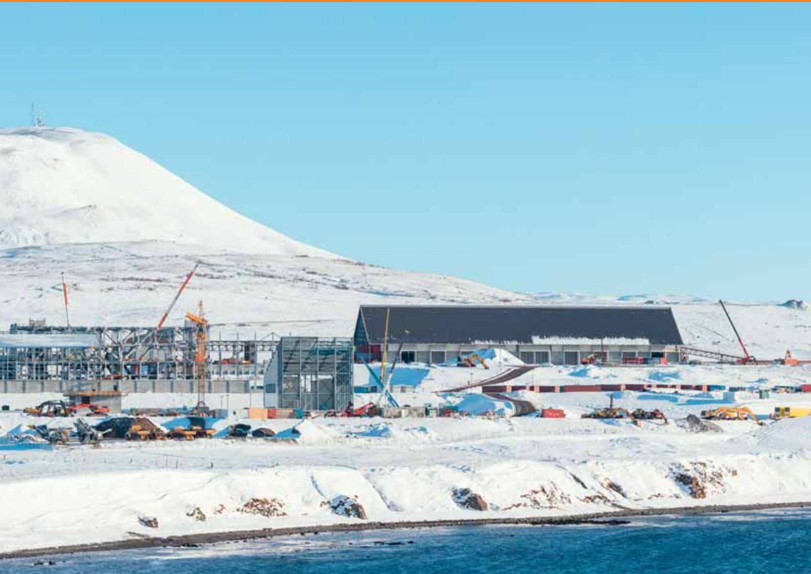
1 Construction work on the silicon metal plant continued unabated even during the winter of 2016/2017, with in particular several cranes working on the central furnace house (centre of photo).
