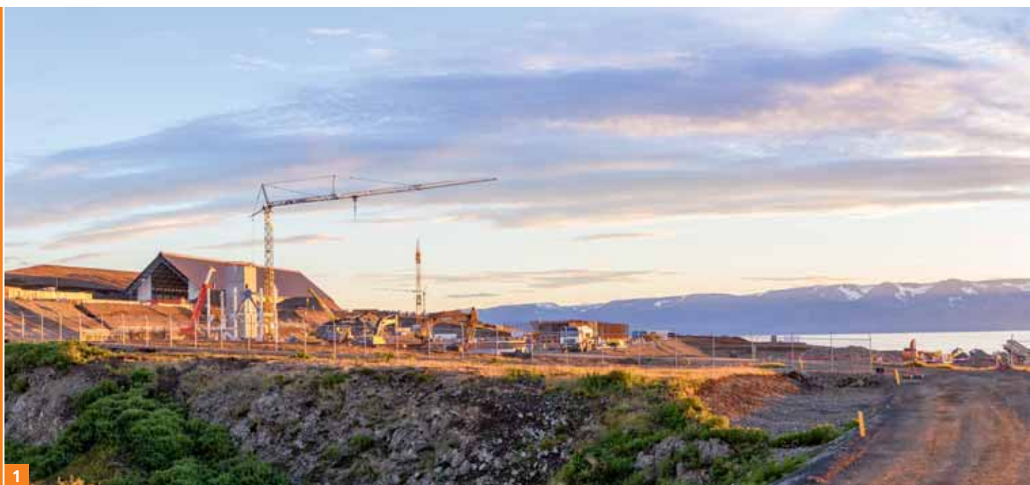
1 The construction site of our silicon metal plant in Iceland. Once completed, the buildings on various terraces will blend perfectly into the landscape.
