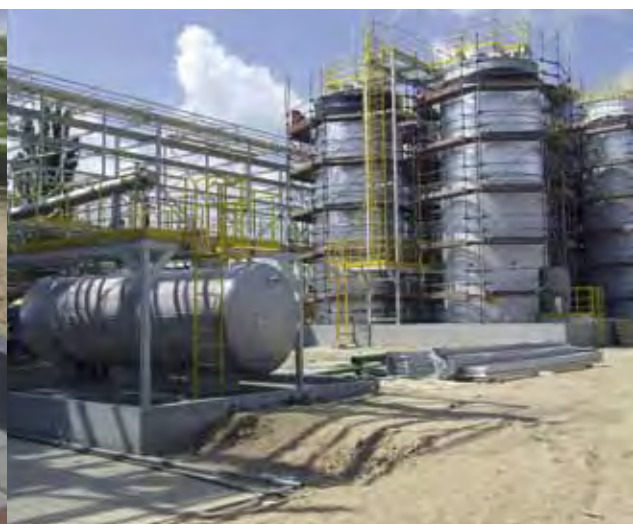
JULY 2010 Buffer tank for ethylene oxide prior to commencement of insulation work
