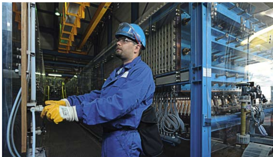
Environmentally friendly membrane electrolysis plant at PCC Rokita SA in Brzeg Dolny.
