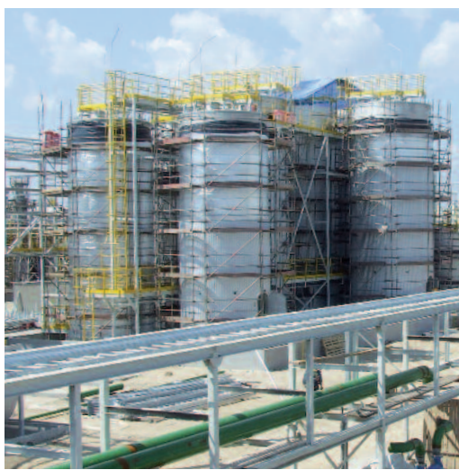
Construction of the fan-assisted cooling towers (left) and the semi-finished and finished product storage tanks (right) of the new ethoxylation plant in Plock, which is scheduled for commissioning at the end of October 2010.
