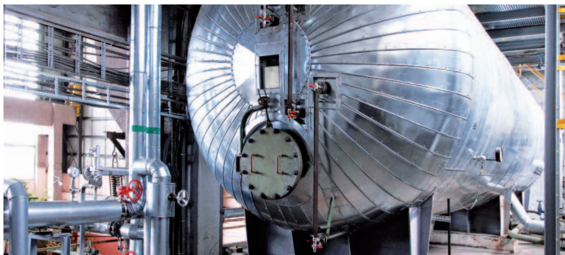
Inside the EC-3 combined heat and power plant, which was connected to the grid at the end of 2008 with a capacity of 14 MW electric and 80 MW thermal.
