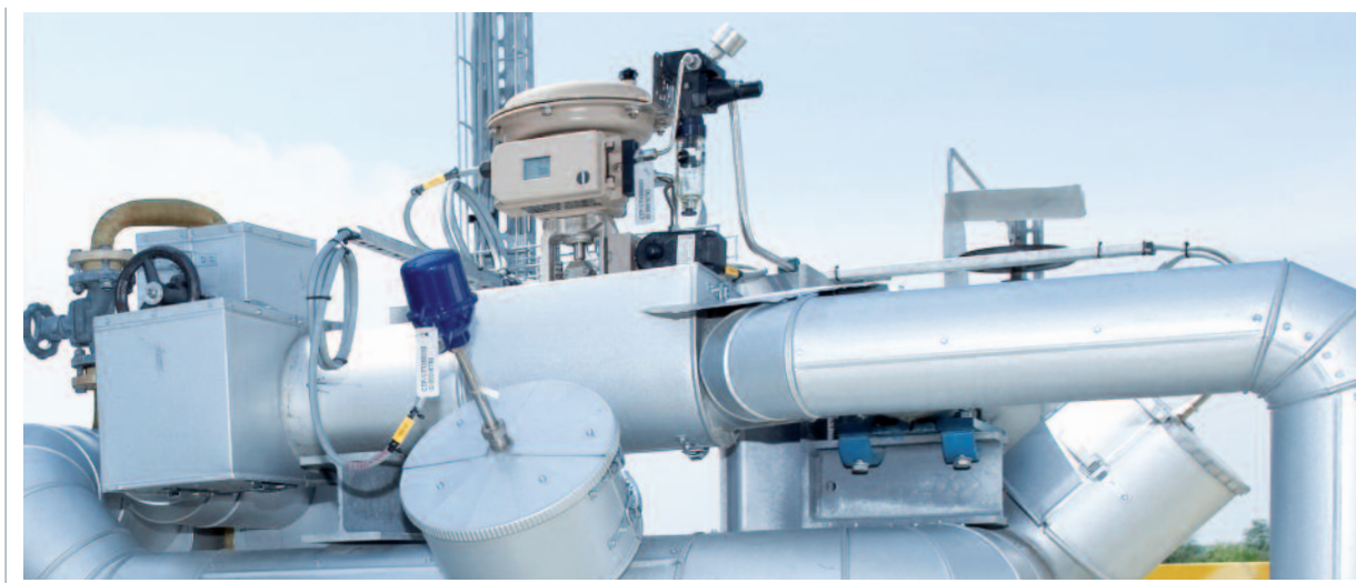
Safety vessels for the chlorine gas system of the membrane electrolysis facility at the site of PCC Rokita SA in Brzeg Dolny.
