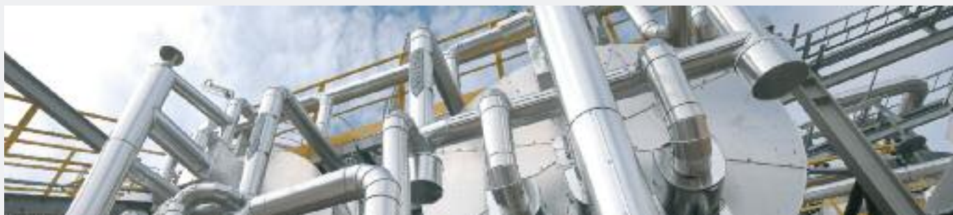
The newly constructed sulphonation plant 2 at PCC Rokita produces around 30,000 metric tons of anionic surfactants per year
