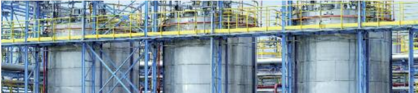
New propylene oxide storage farm of PCC Rokita – three tanks with a volume of 160 cubic metres each
