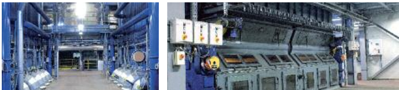
The new CHP plant EC-3 is a coal- and biomass-fired cogeneration facility boasting state-of-the-art technology
