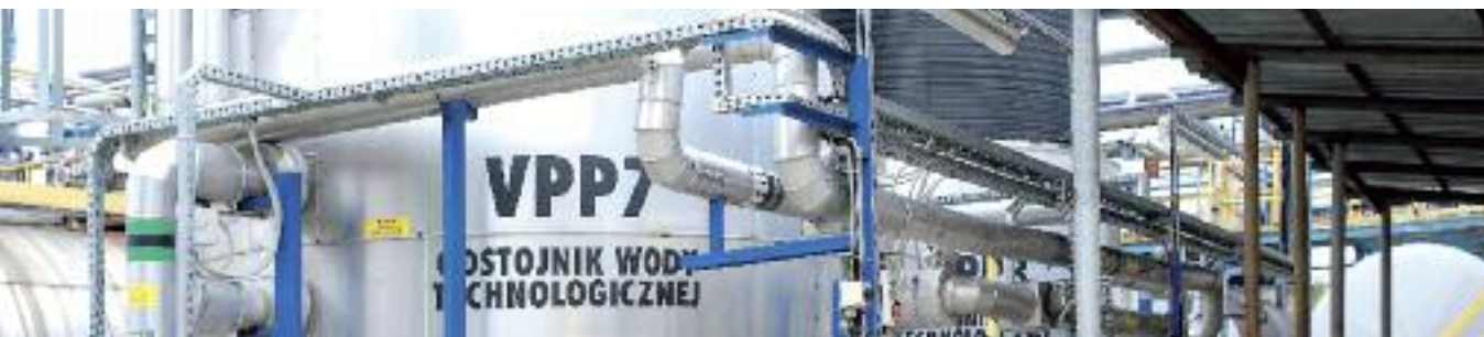
New process water settling tank for the Phosphorus Chemicals business unit at PCC Rokita
