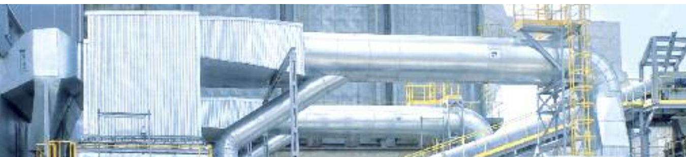
The combined heat and power plant EC-3 on the site of PCC Rokita in Brzeg Dolny was commissioned in October 2008
