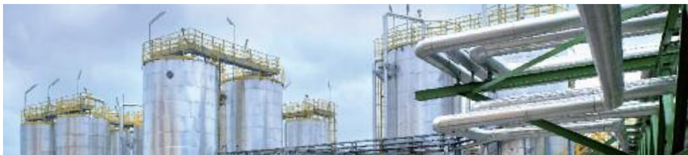
Storage tanks at the new sulphonation plant of PCC Rokita in Brzeg Dolny – commissioned in 2008
