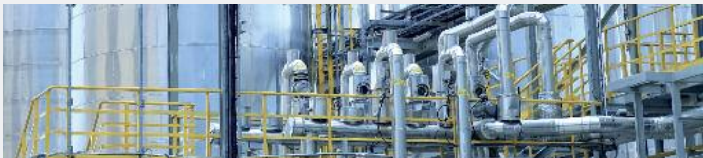
PCC Rokita is the only manufacturer of surfactants in Poland – here its new sulphonation plant 2 for the production of the anionic surfactants
