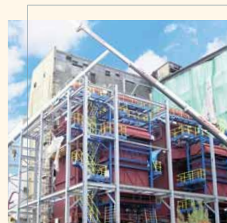
The new combined heat and power plant of PCC Rokita will ensure the supply of, among other things, district heating to the approx. 14,000 inhabitants of Brzeg Dolny
