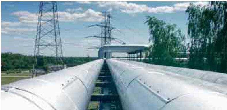
Piping system on the factory site of PCC Rokita
