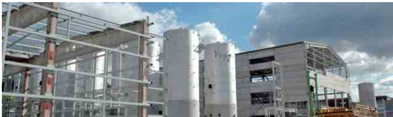
Structural framework of a new sulphonation plant at PCC Rokita scheduled for completion by the end of 2007
