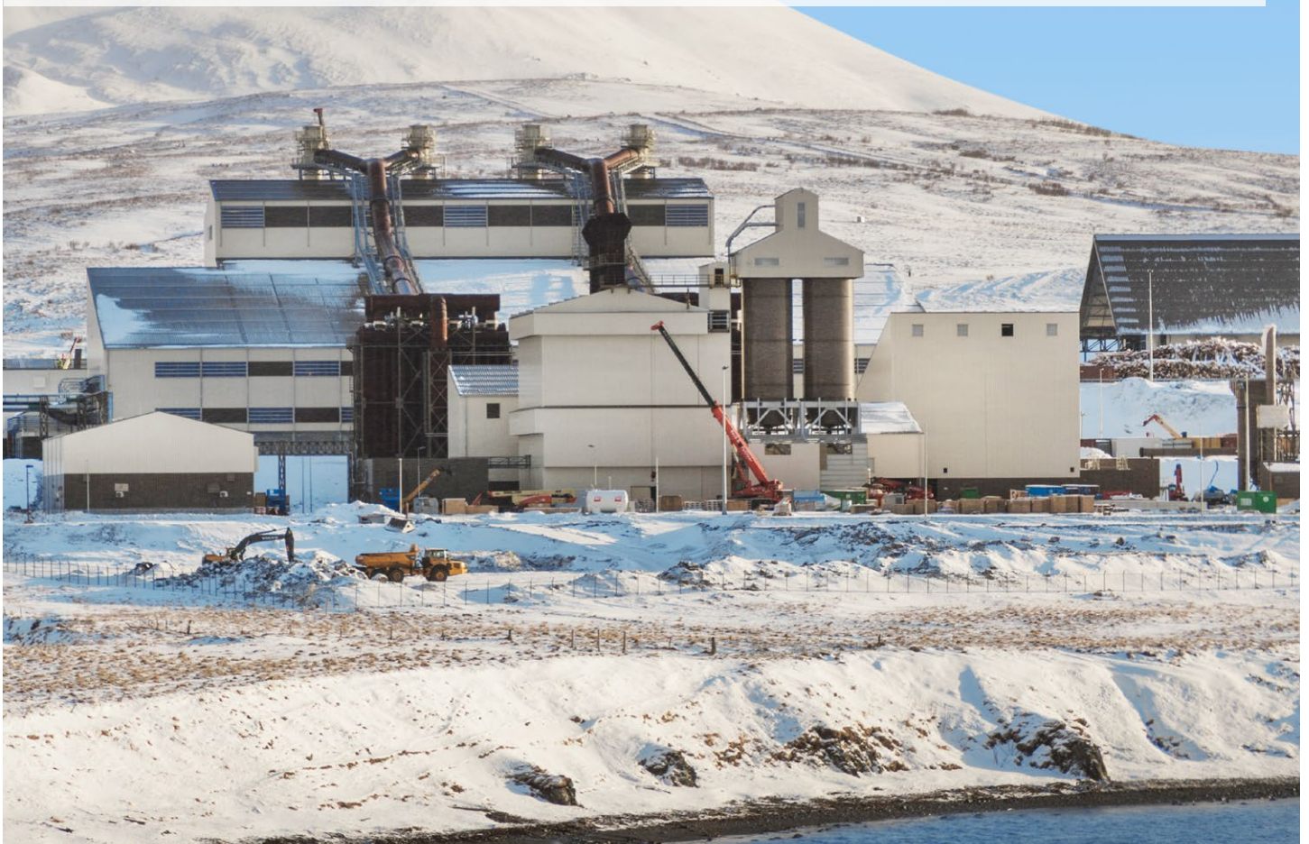
Construction site of PCC BakkiSilicon hf in the north of Iceland in February 2018: In the center background can be seen the building containing the two electric arc furnaces. Commissioning is scheduled for the end of March / beginning of April, 2018.
