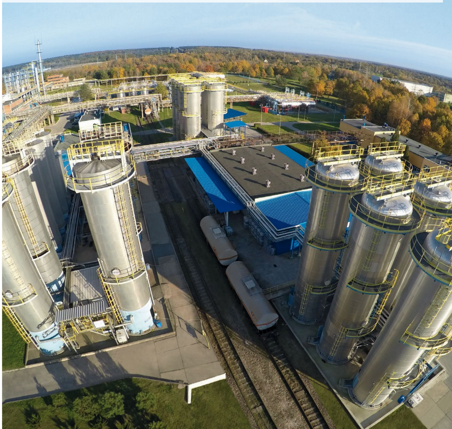
Part of the tank farm for polyols with filling station for drums and intermediate bulk containers (IBC) at the site of PCC Rokita in Brzeg Dolny (Poland)
