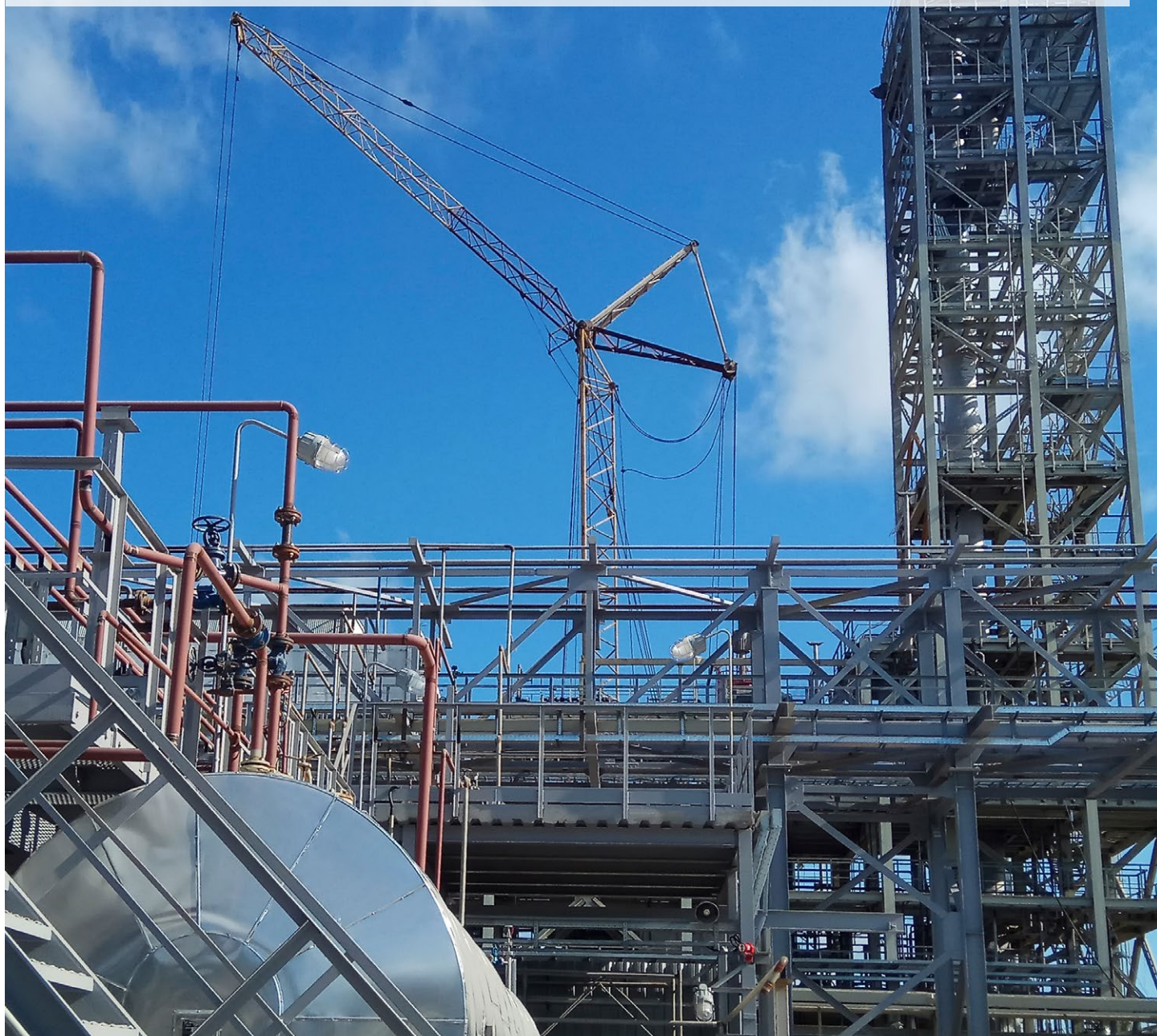
The production plant for high-purity aerosol-grade dimethyl ether (DME) of our Russian joint venture DME Aerosol, Pervomaysky, as of August 2018. Commissioning is scheduled for fall 2018. Pictured right is the approx. 45 meter high distillation column.
