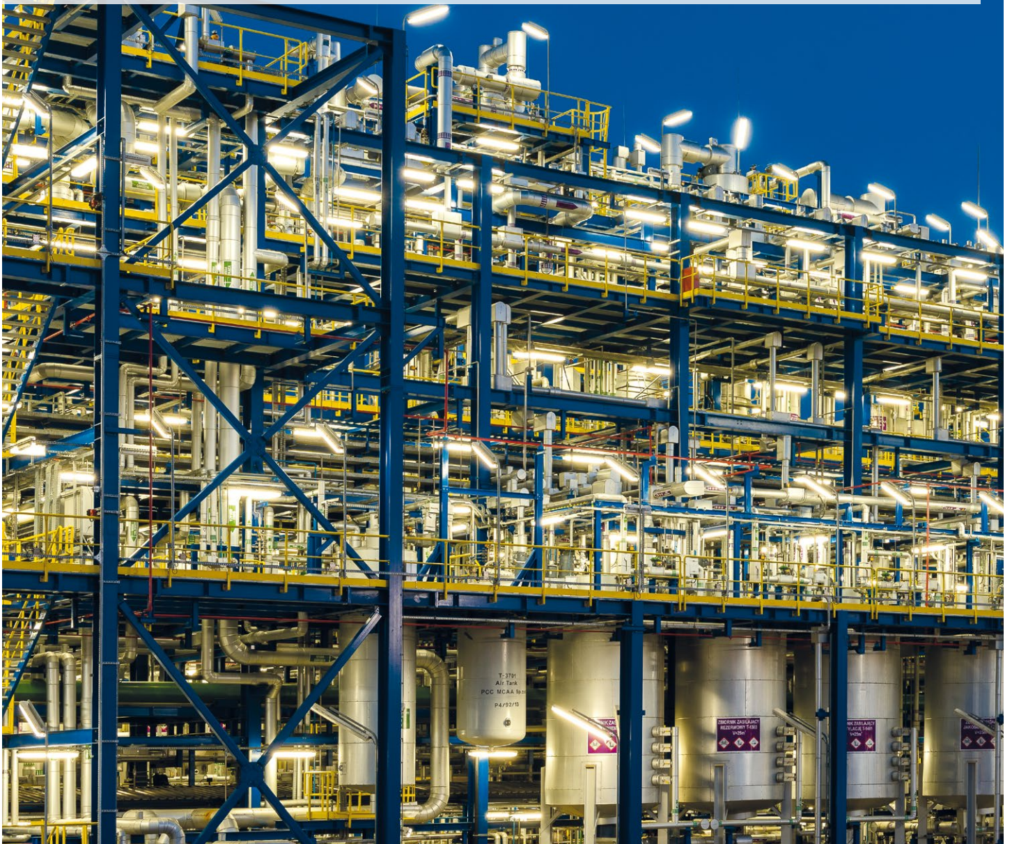
New production plant for monochloroacetic acid (MCAA) operated by PCC MCAA Sp. z o.o. in Brzeg Dolny (Poland): The facility significantly extends the chlorine value chain of the PCC Group. It also facilitates backward integration, as MCAA can be used as a feedstock for betaine production in our Surfactants segment.
